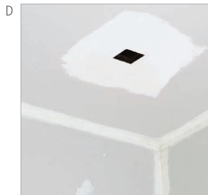
Skim coat around the plaster plate and up to the aperture for a seamless appearance.
